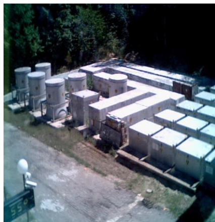
Fig.22 Temporary structures for storage of spent sealed radioactive sources, consisting of five reinforced concrete container type "PEC".
