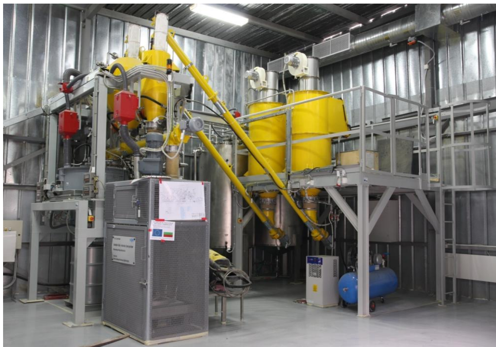
Fig.9 Cementation unit for conditioning of low level radioactive waste
