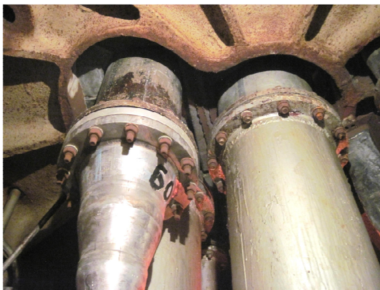
Figure 4. Flanges to the reactor vessel.
